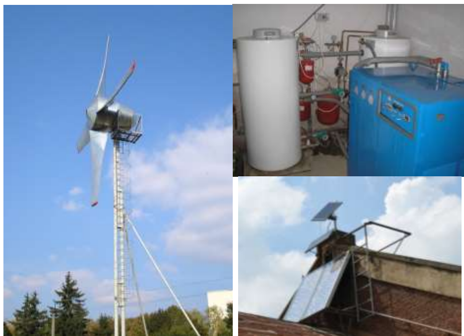
Fig. 5. General view of components of the hybrid system of power supply of a laboratory RSE
